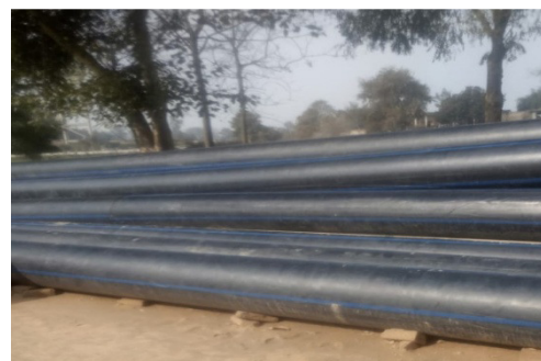
Pipes lying in Chuharia village
